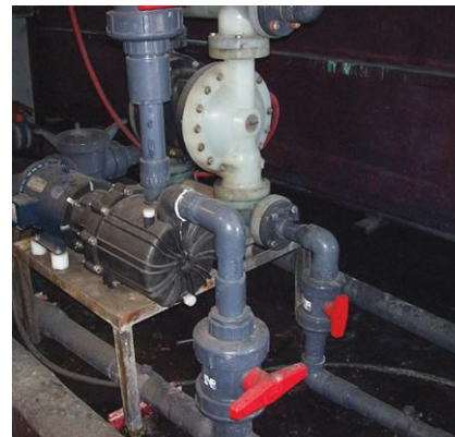
IMAGE 6: Electric self-priming pump replacing AODD pumps
