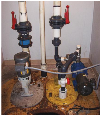
IMAGE 4: Self-priming pump replacing in-solution vertical pump
