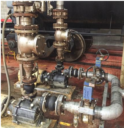
IMAGE 3: Self-priming pumps used to unload rail tanker cars
