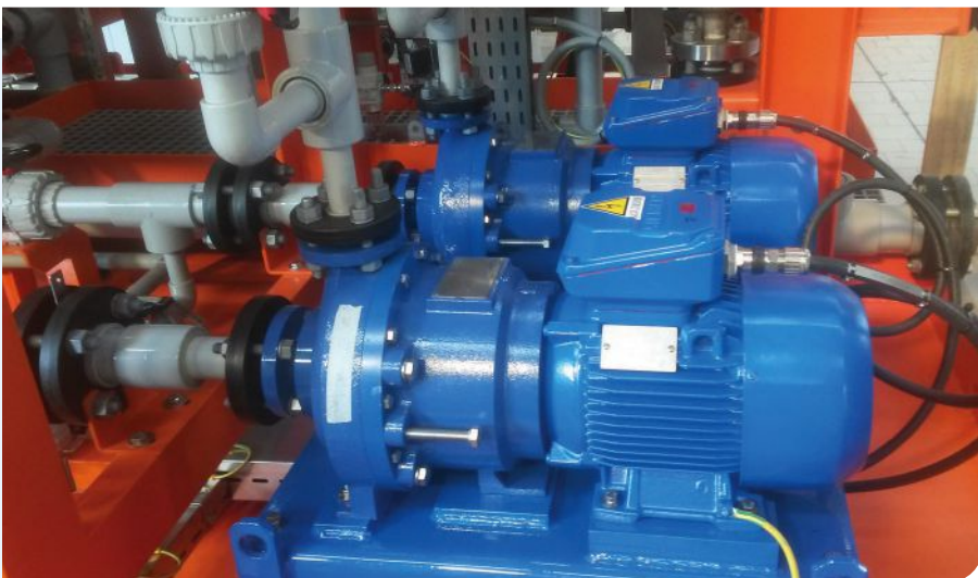
FIGURE 2: Finish Thompson ULTRAChem pumps installed in an electrochlorination system, in which sodium hypochlorite is produced from running saltwater through electrolytic cells. It's for use in the water and waste water treatment industry. Courtesy Finish Thompson
